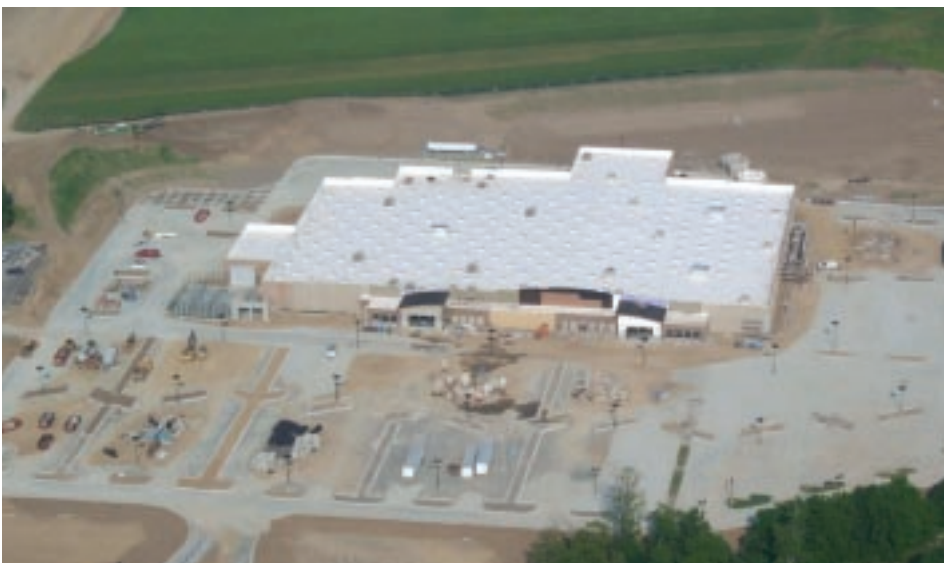
▲ Schlouch crews cover the landscape as they continue work on the 63-acre site for Walmart in Tunkhannock, Wyoming County, PA.
