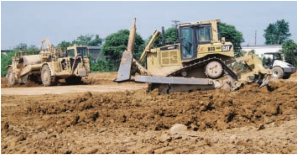
▲ Schlouch's heavy equipment displays its power as it constructs a site for a Bottom Dollar food store in Nazareth, Northampton County. The 4-acre site is one of two sites in the Lehigh Valley where Schlouch is providing sitework for Bottom Dollar projects. (continued from page 3)
