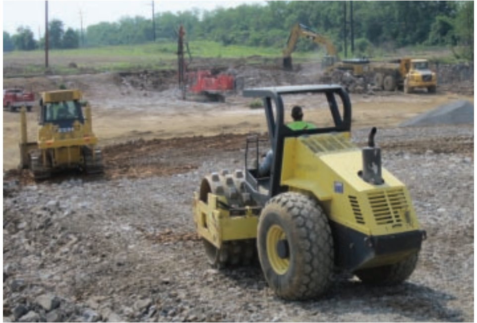
▲ Once again working with Tippmann Construction, Schlouch is preparing a 40-acre site for a Giant Foods perishable distribution center in Cumberland County, PA.
