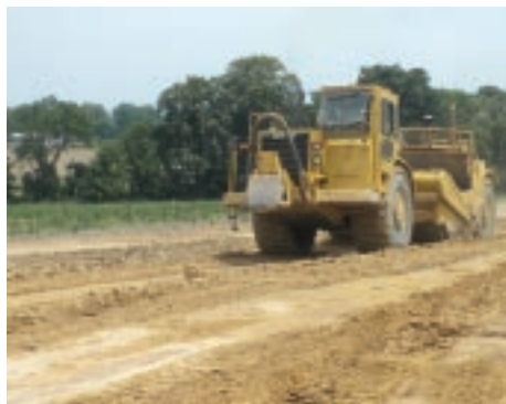
▲ A scraper at Trexler Fields begins roadway preparation on a residential site for 10 twin homes and 21 single-family homes.
