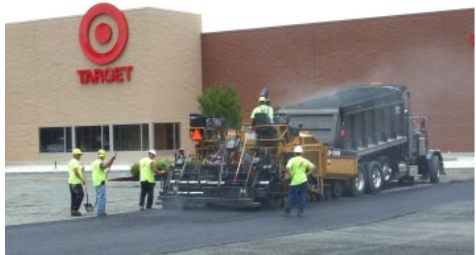
▲ Schlouch asphalt paving crew begins paving of parking area at the Target facility in the Newman Reading Associates project on 5th Street Highway, Muhlenberg Township, Berks County. In addition to Target the center will feature Giant Foods, PetSmart and a bank.
